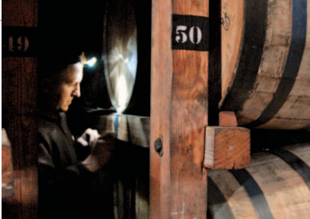
Working by the light of his headlamp, Quinn scrapes a leak smooth to ready it for repair.
